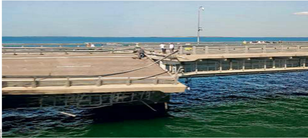
A still image from video showed a section of the bridge split and listing to one side in the aftermath of the attack.
