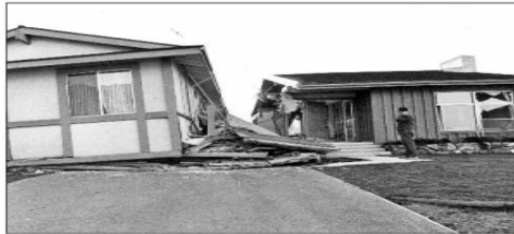
A HOME was destroyed in the 1971 Sylmar earthquake when the second story collapsed on its garage.
