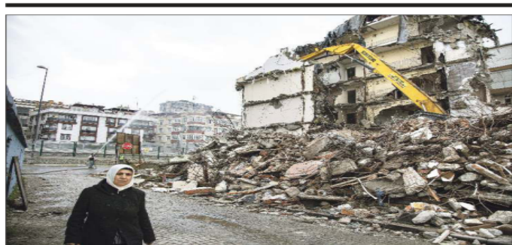
RESMA EFFENDI For The Times A BUILDING in Istanbul undergoes demolition on the day a family from an adjacent block moved from the apartment they owned into a rented home.
