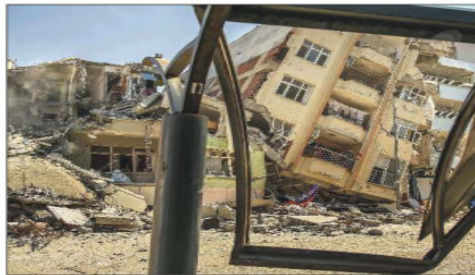
MANY of the concrete buildings that collapsed in last month's earthquakes had inadequate reinforcing.
